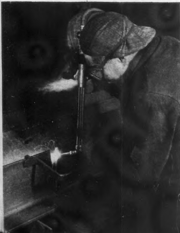
FIG. 6 —The V-notches cut in the bottom members while on the beam splitting table are hand torch beveled preparatory to bending and welding. A removable arm rest is employed for steadying the operator's guiding hand. This job is done in transit.
